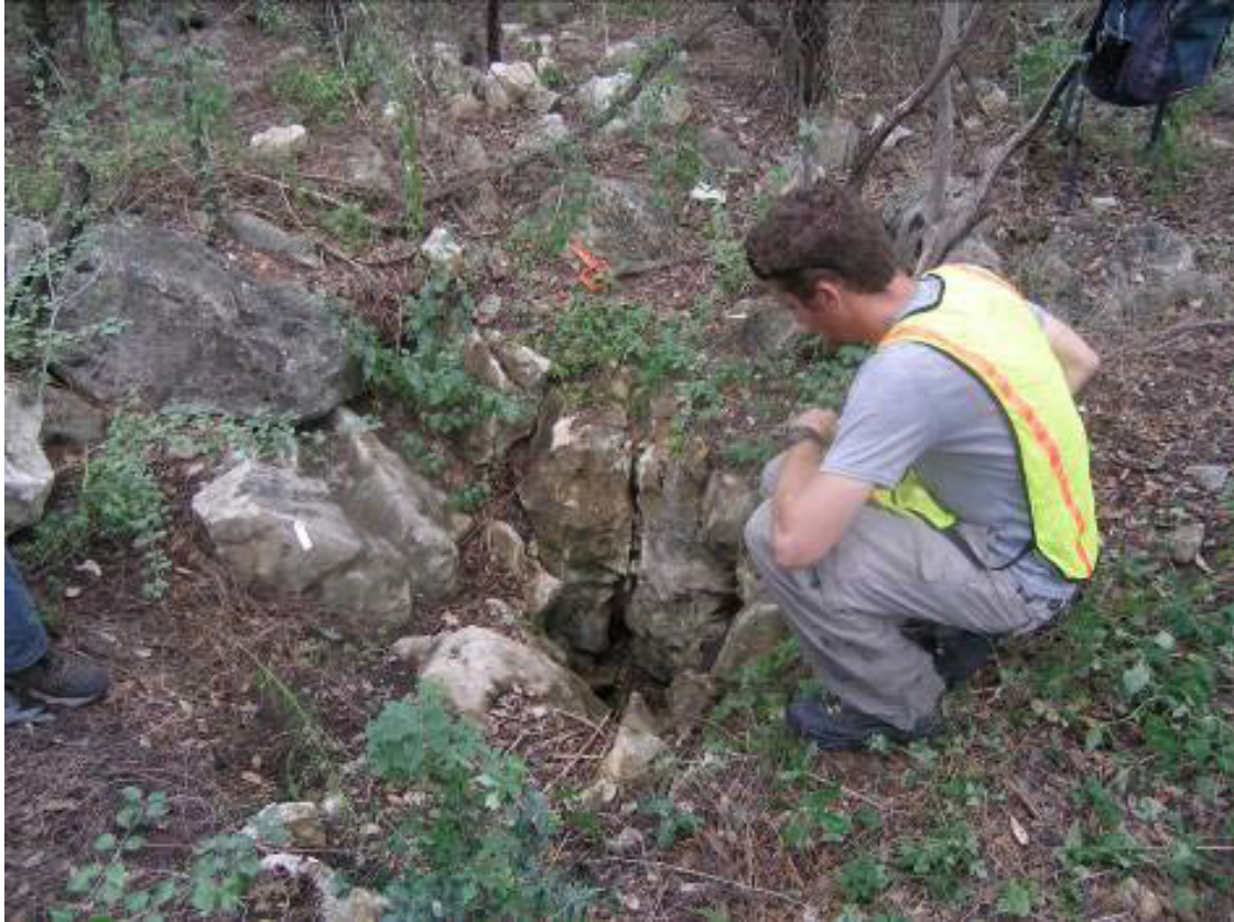
This sinkhole measures 9 ft in diameter and 12 ft in depth. It receives flow from approximately 10 square meters off a hilltop.
