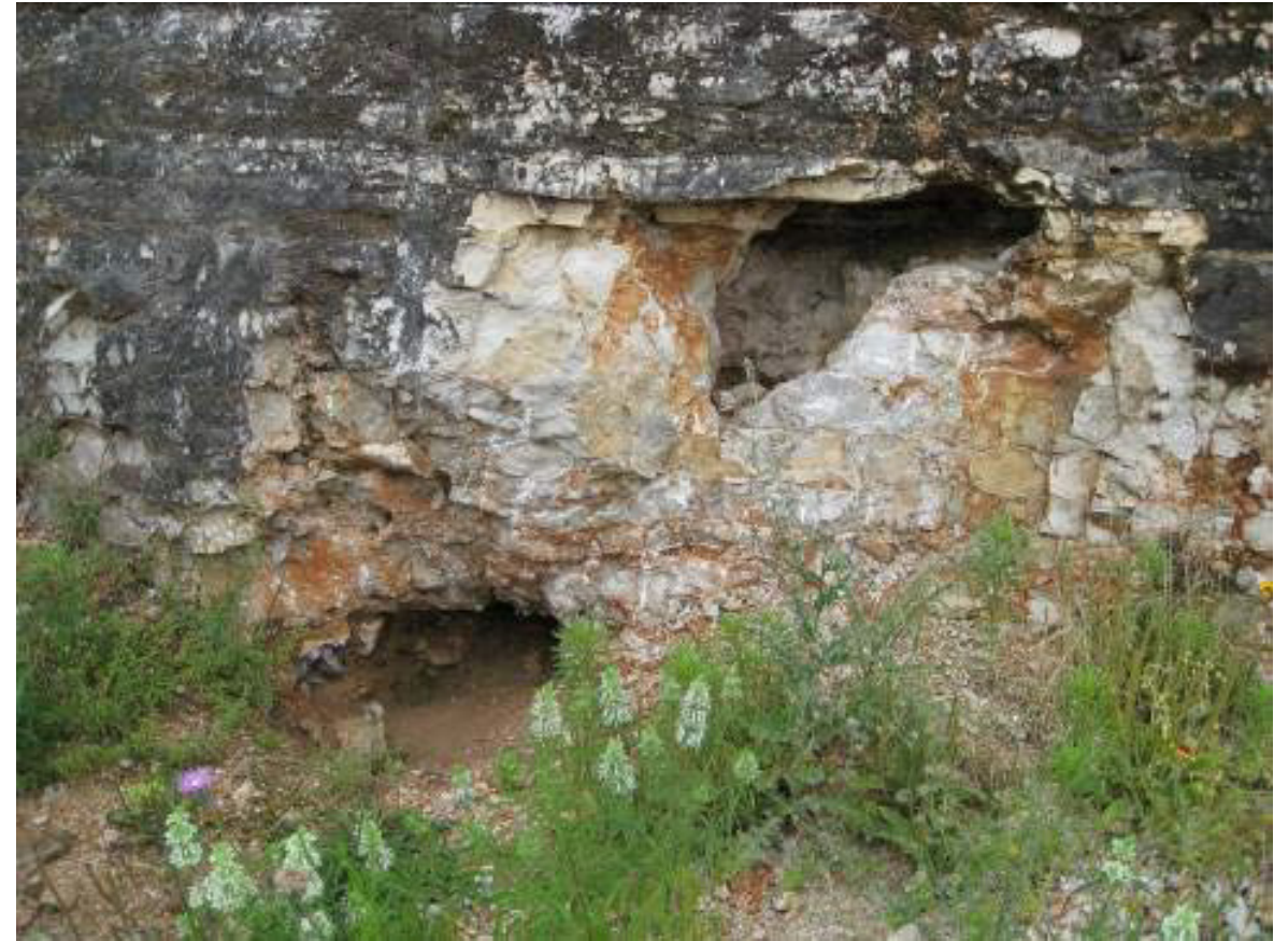
This cavity consists of an upper and lower void joined together by a shaft measuring 2 ft wide, extending 1.5 ft into a roadcut face, and 3.3 ft in total height.
