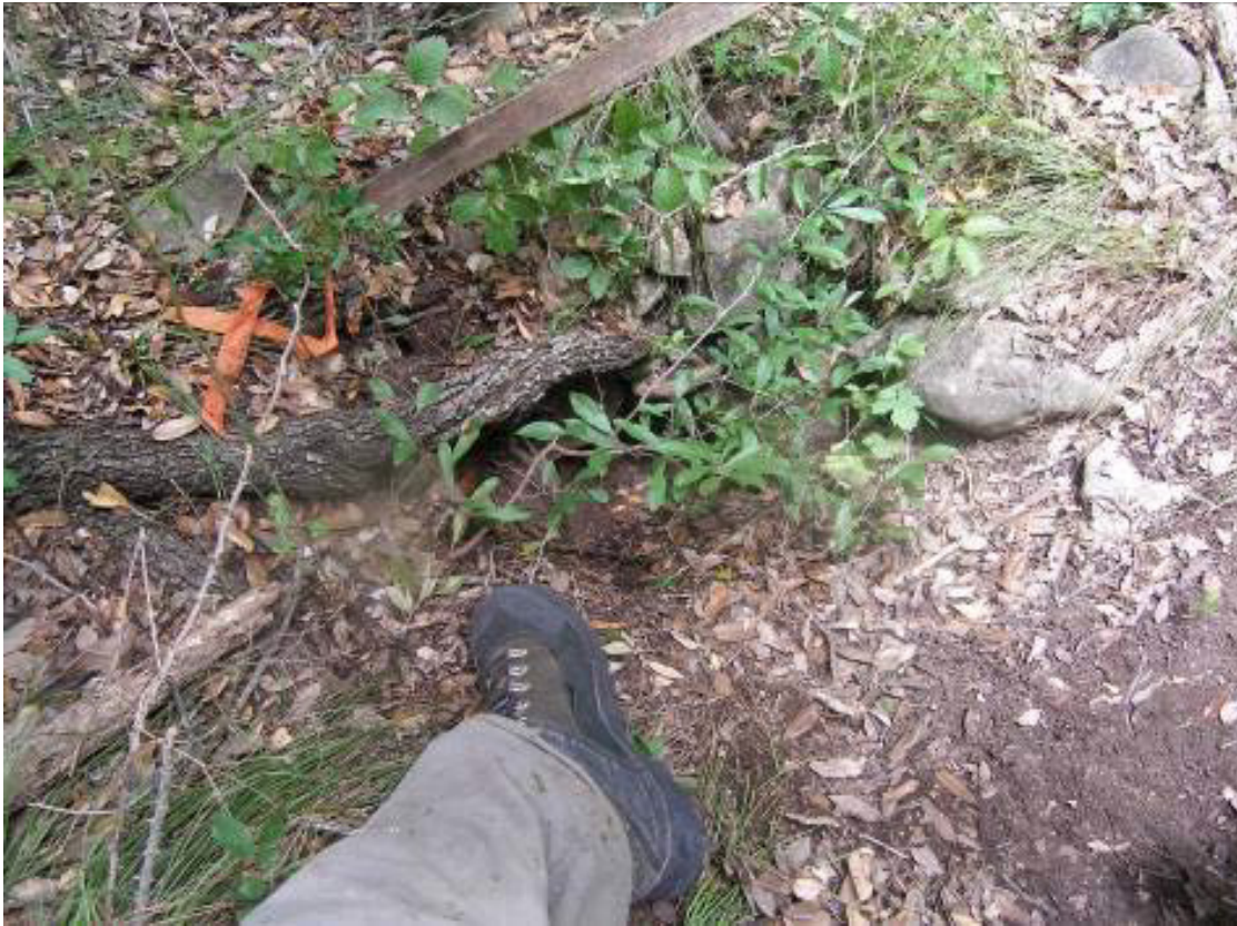
This sinkhole measures 4.6 ft in diameter and 3 ft in depth. It appears to have a drain continuing further underground out of sight and out of reach
